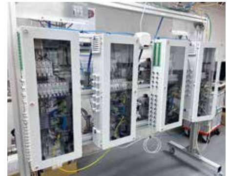
Fig. 10: Control boxes for connecting flange heating and temperature sensors to the DIPAK test vessel.
