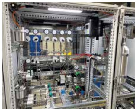
Fig. 9: Multi-channel gas mix- and gas analysing system for the DIPAK gas supply infrastructure.
