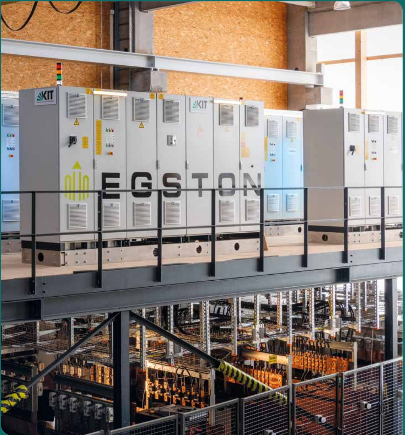
Power Hardware In the Loop testing hall
